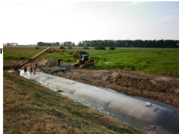
Photo 3 . Initial stage of filling the geotextile tube by sand and water mixture, Photo by Huesker
