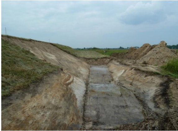
Photo 1 . Excavation at dike toe, prepared for installation of geotextile tube, Photo by Huesker
