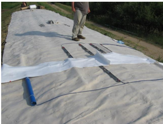
Photo 2 . Geotextile tube SoilTain ® monitoring system by Neostrain ® , Photo by Inora
