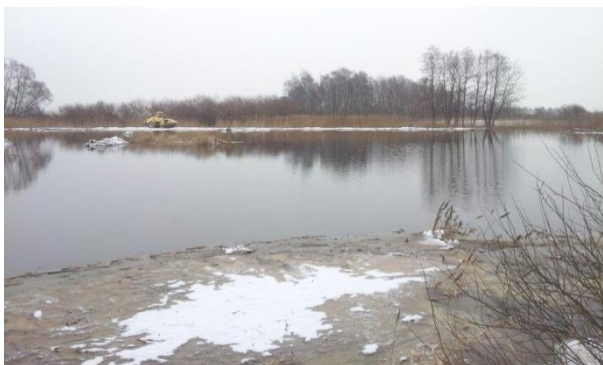
Fig. 9. Flooded construction site 01-2014
