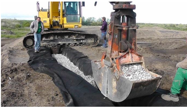
Fig. 4. Installation of the rigole, connected to a geosynthetic drainage composite to control the phreatic level
