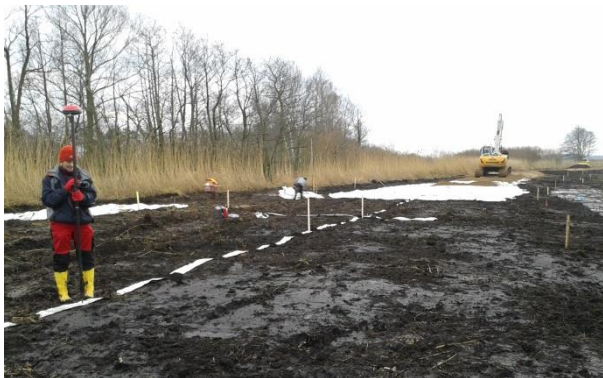
Fig. 8. Construction of the dike core on geosynthetic and wire placement underneath the dike 12-2013
